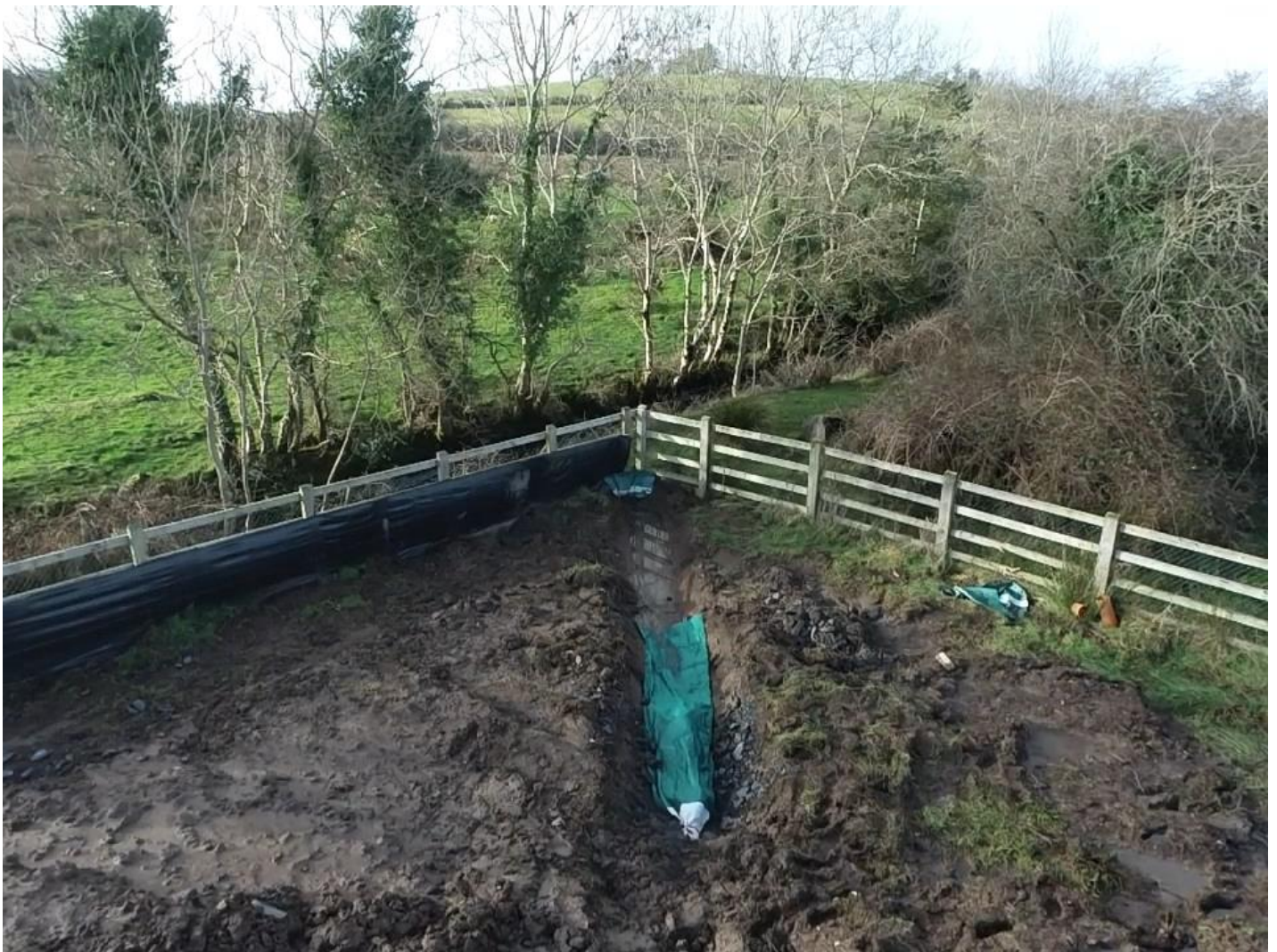
Figure 7-22 Example of a Silt Sock placed on the outlet pipe
